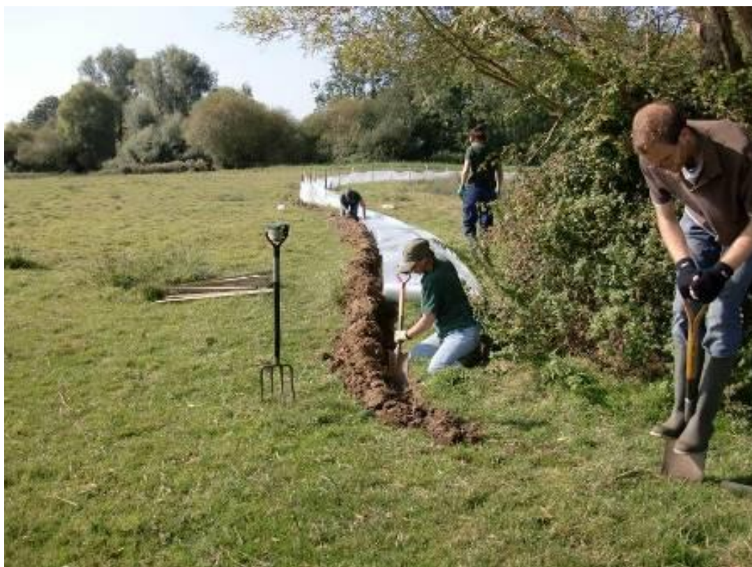
Figure 98: Wildlife Trust staff and volunteers installing the fence around Round Pond (Photograph: Sarah Jackson)
