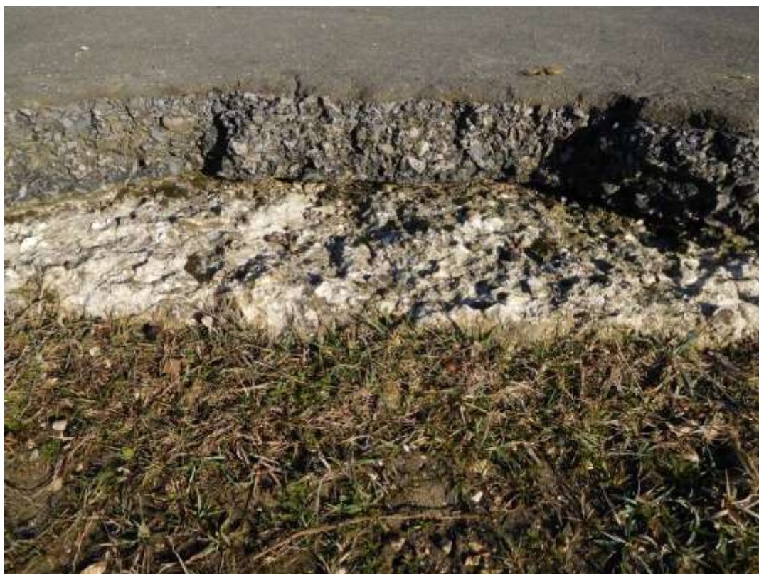
Figure 15: A cross-section through the perimeter road of the former airfield at Beaulieu Heath showing concrete underlying the tarmac. Photograph taken on 28 November 2016.
